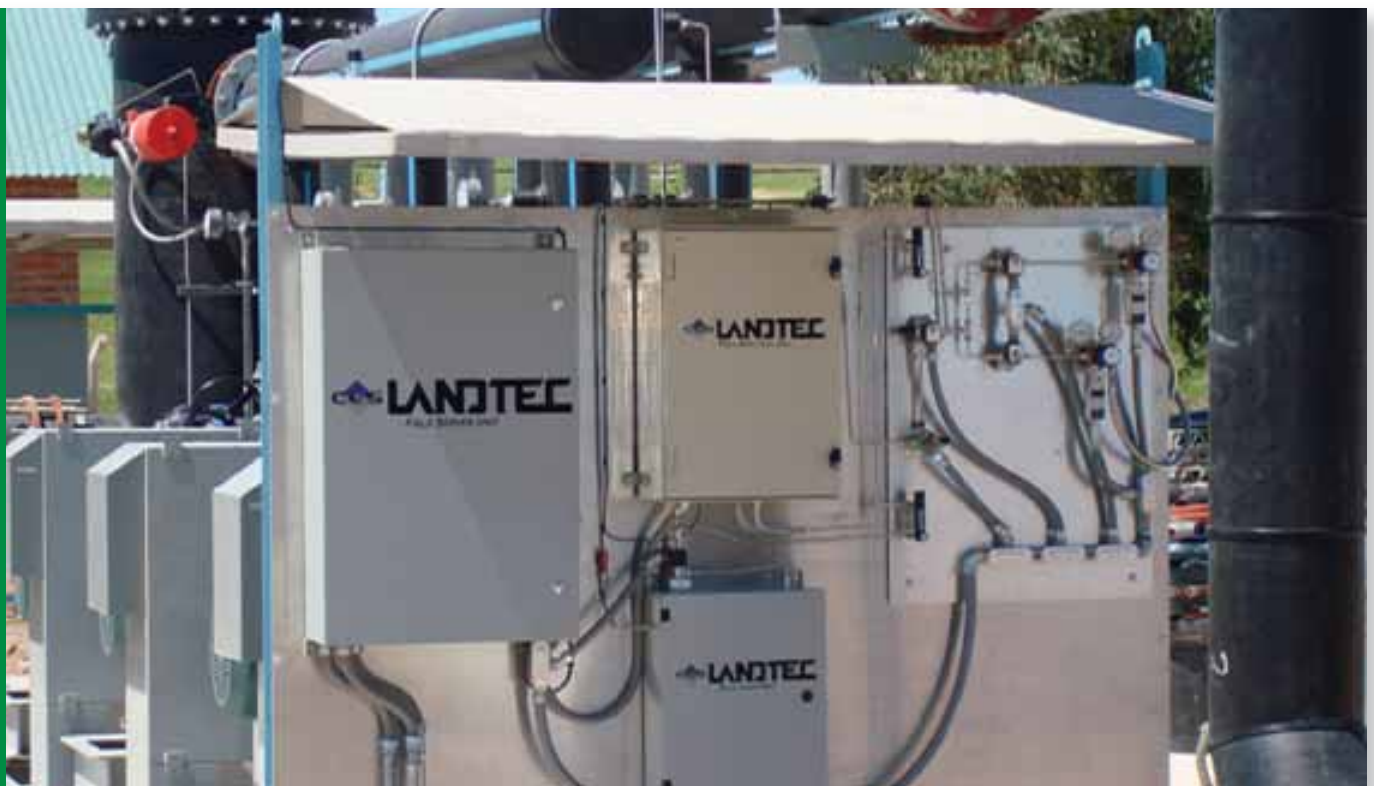
Unmanned and Remote, Automatic Extraction Monitoring System Equipment at Work
