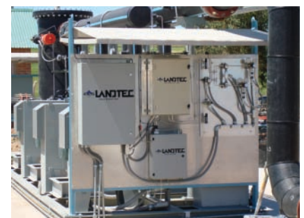
Automated landfill gas extraction monitoring system
