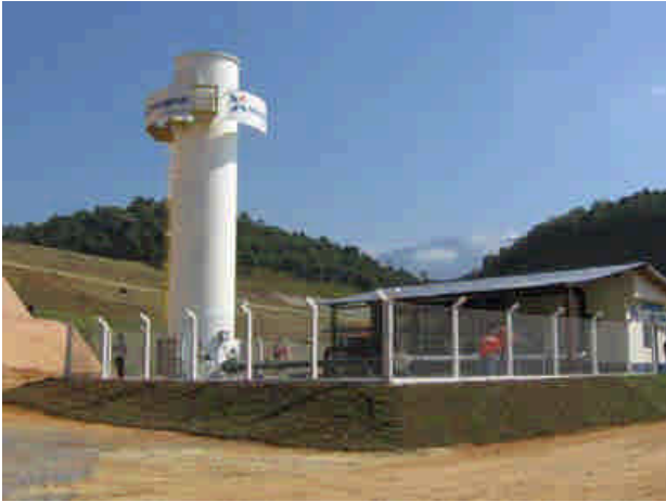
FLARE STATION (Novagerar monitoring report 2008)
