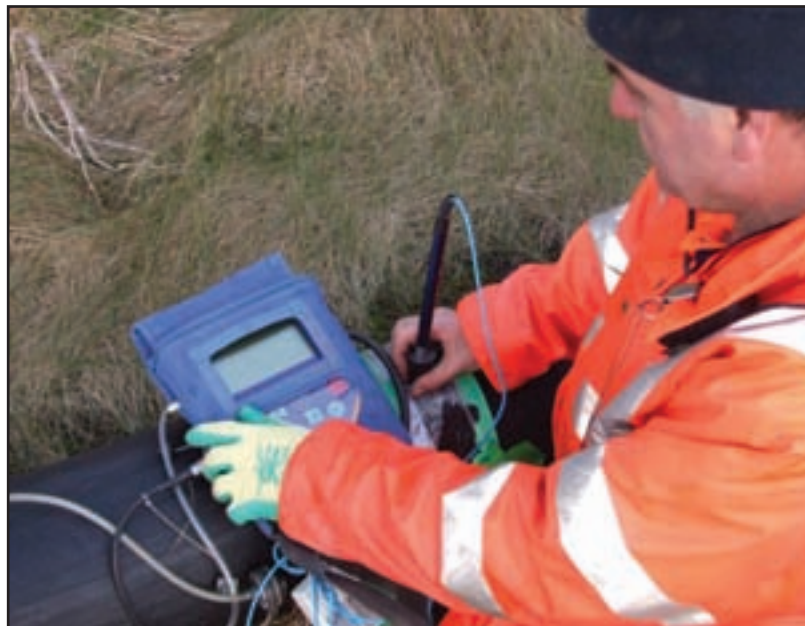
A GA2000 portable landfill gas analyser is used to check gas quality, pressure and flow
